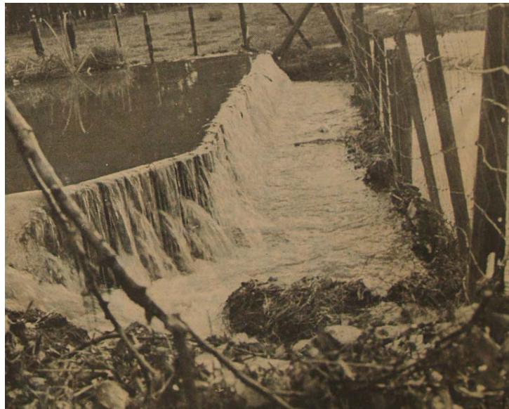
Image 5.9: Malfunctioning stormwater rubbish trap, February 1977 1184
